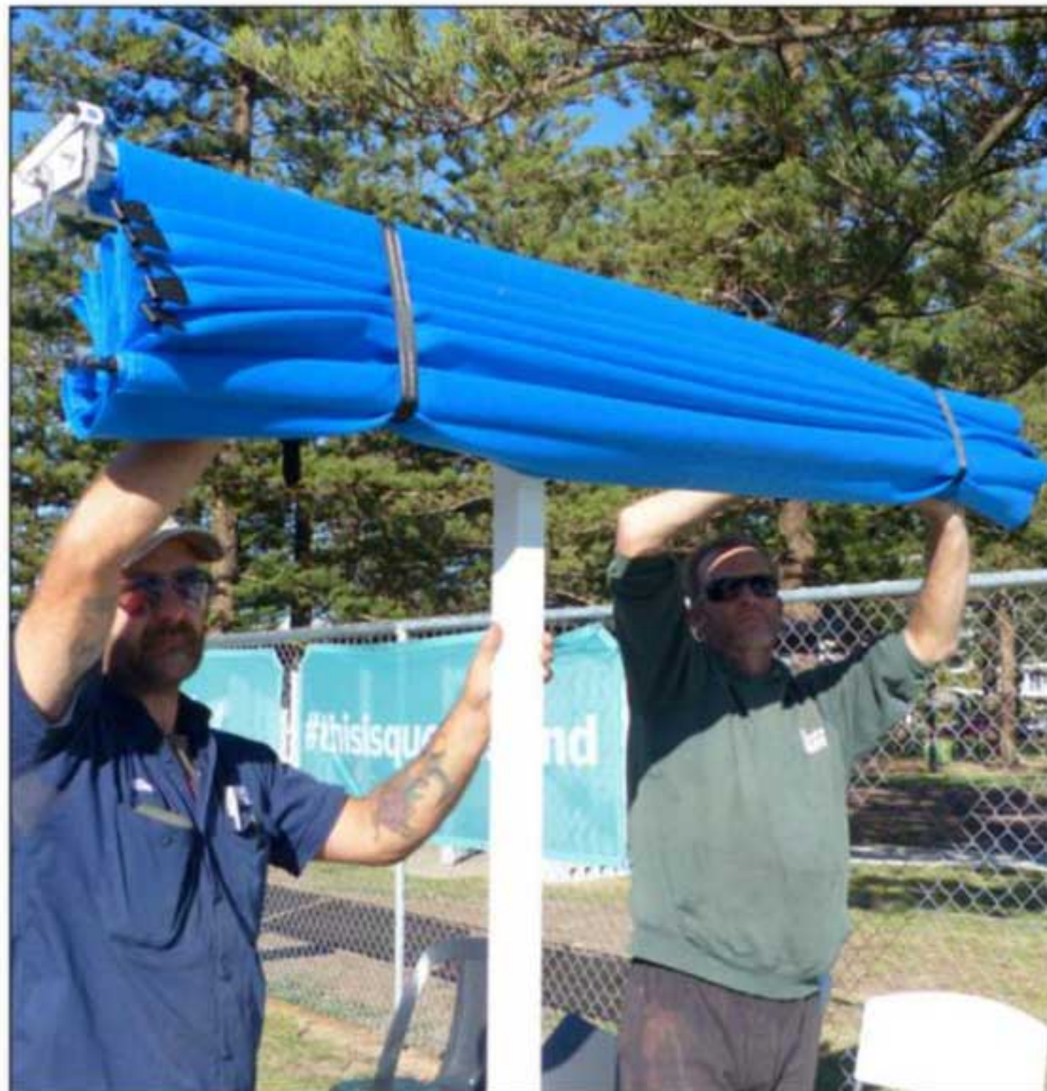
• Shadex technicians ensure every aspect of the installation adheres to a strict best practice criteria.
